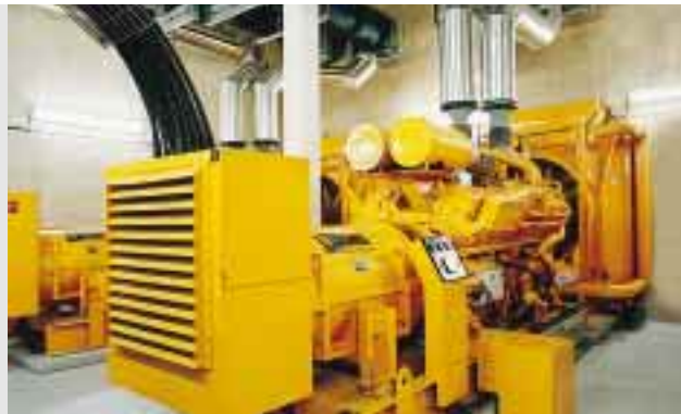
2x1600kVA medium voltage generating sets with paralleling
