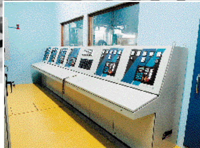
Sound-proofed control and management room
