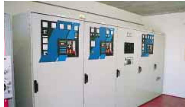
Sound-proofed control and management room
