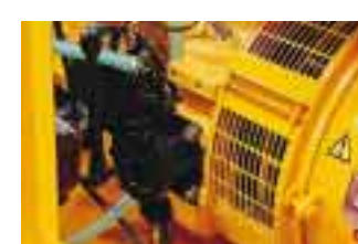
Sump drain pump (to MS130SiL)
