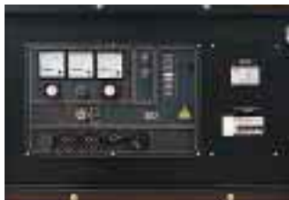
Control breaker on front panel
