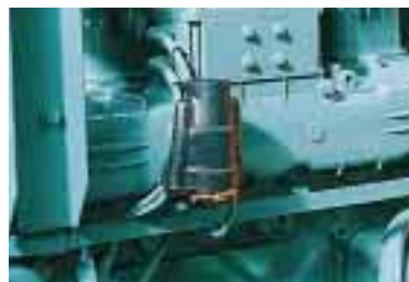
Air heater (intake pre-heating)
